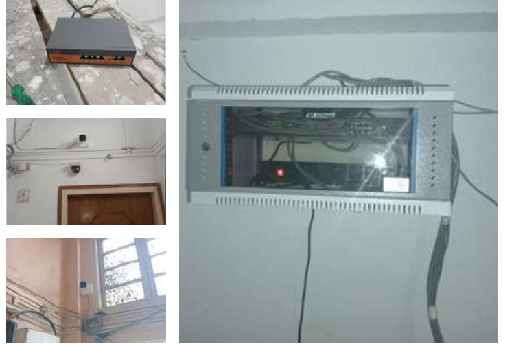
AIIDC - DOME AND BULLET CAMERA INSTALLATION AIIDC OFFICE BUILDING INDOOR & OUTDOOR
