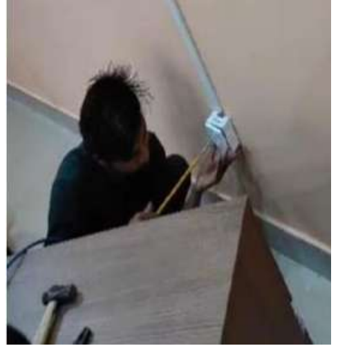
TEZPUR DATA CENTER
